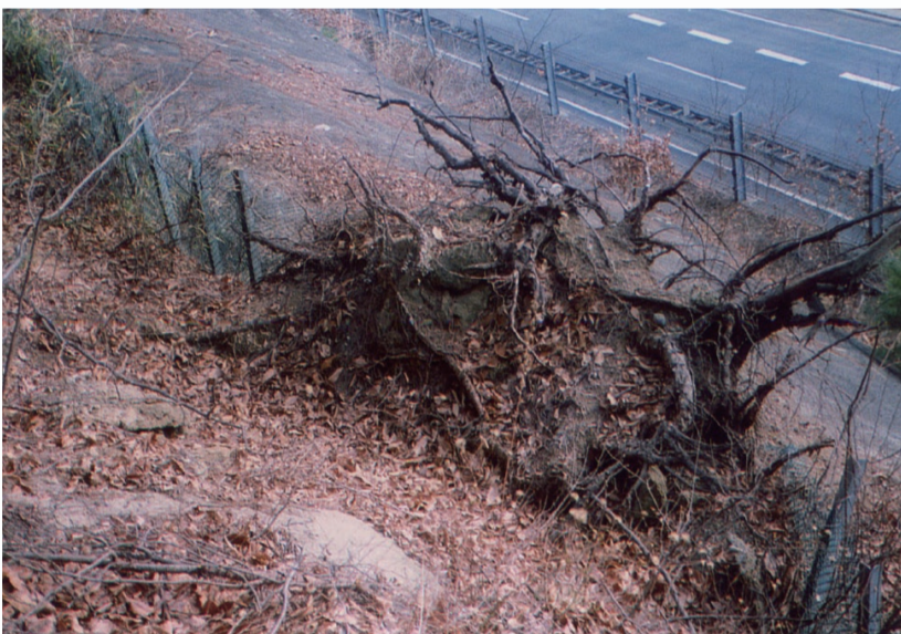
切土のり面の倒木
